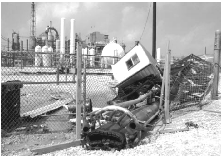
Figure 4.1.14 Flare Tower Damage – Hurricane Rita (Photo Courtesy of FEMA)
