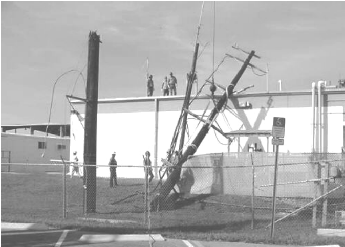
Figure 4.1.4 Power Pole – Hurricane Frances (Photo Courtesy of NASA KSC)
