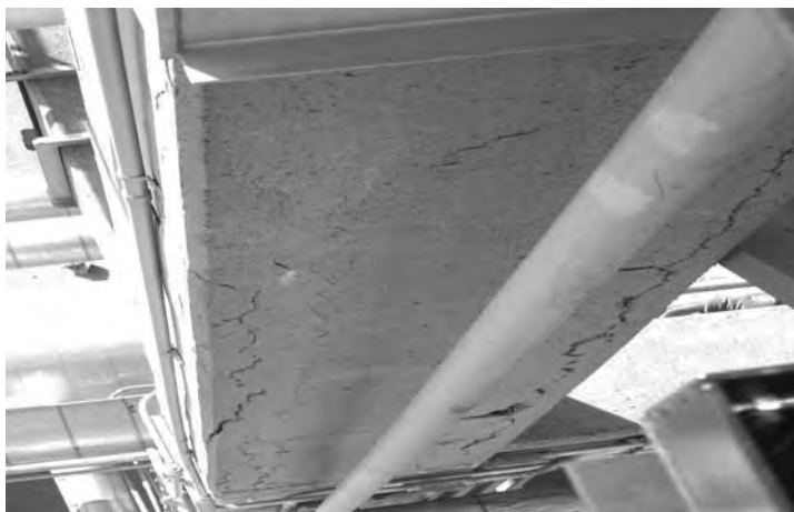
Figure 4.6.3 Photo of Deterioration of a Concrete Column
