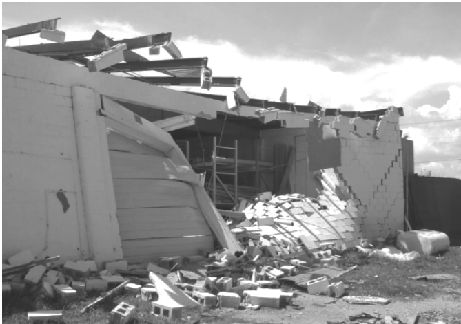
Figure 4.1.3 Building with Masonry Infill – Hurricane Charley
