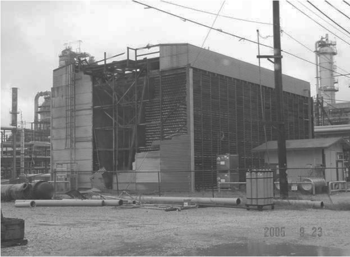
Figure 4.1.19 Cooling Tower Damage – Hurricane Rita (Photo Courtesy of Louisiana Chemical Association)
