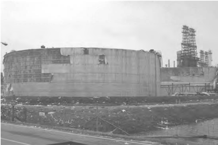
Figure 4.1.12 Tank Cladding Damage – Hurricane Rita (Photo Courtesy of Louisiana Chemical Association)
