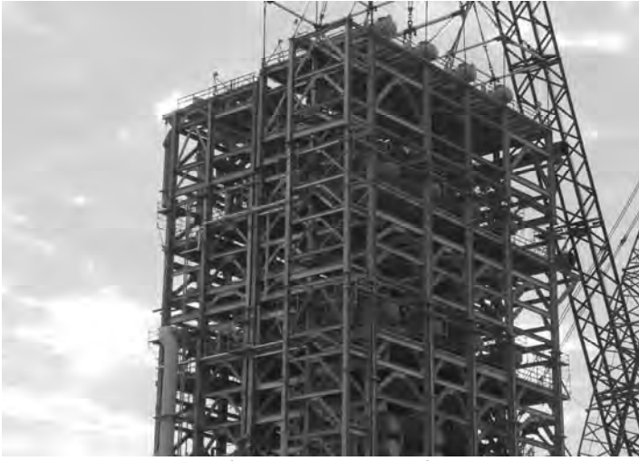
Figure 5B.1 Typical Process Structure with Dense Arrangement of Equipment and Piping
