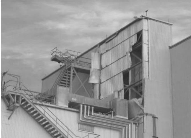
Figure 4.1.6 Cladding Damage – Hurricane Frances (Photo Courtesy of NASA KSC)
