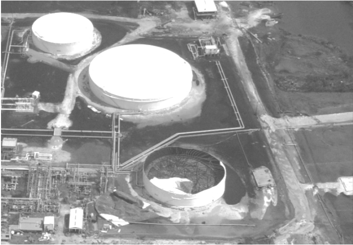
Figure 4.1.9 Tank Damage - Hurricane Katrina (Photo Courtesy of NOAA)
