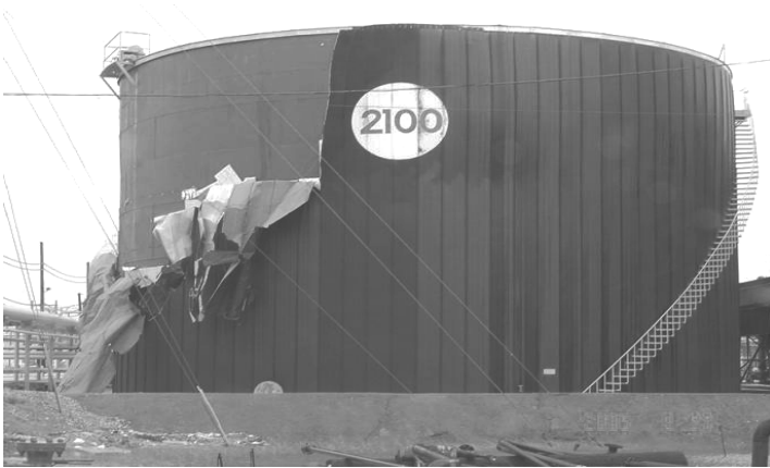
Figure 4.1.13 Tank Insulation and Cladding Damage – Hurricane Rita (Photo Courtesy of Louisiana Chemical Association)
